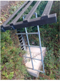
1. Broomhouse Lane, Edlington Trash Screen Checked before any predicted heavy rainfall events to assess requirement for cleansing.
