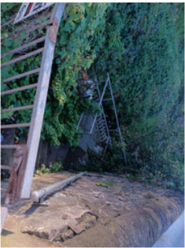
1. Sheffield Road, Conisbrough Trash Screen Checked before any predicted heavy rainfall events to assess requirement for cleaning.
